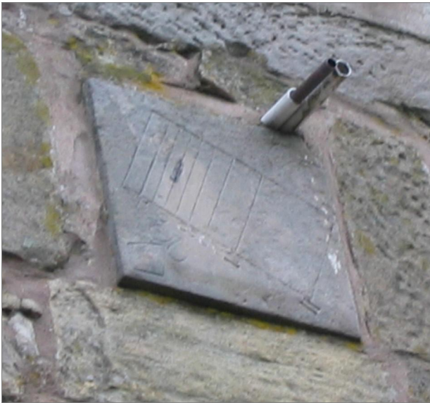
Fig. 5. Preston Lodge's east facing sundial complete with overflow pipes.
