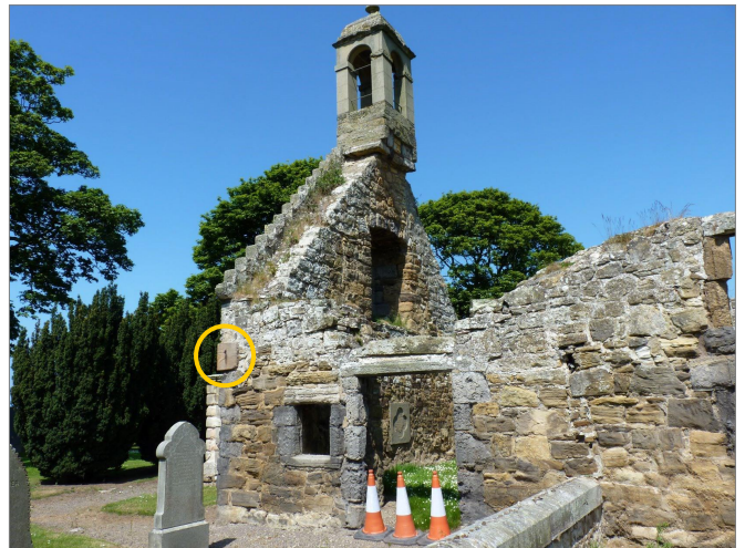
Fig. 11. The Gladsmuir sundial today (circled) with the precarious-looking bell tower behind.
