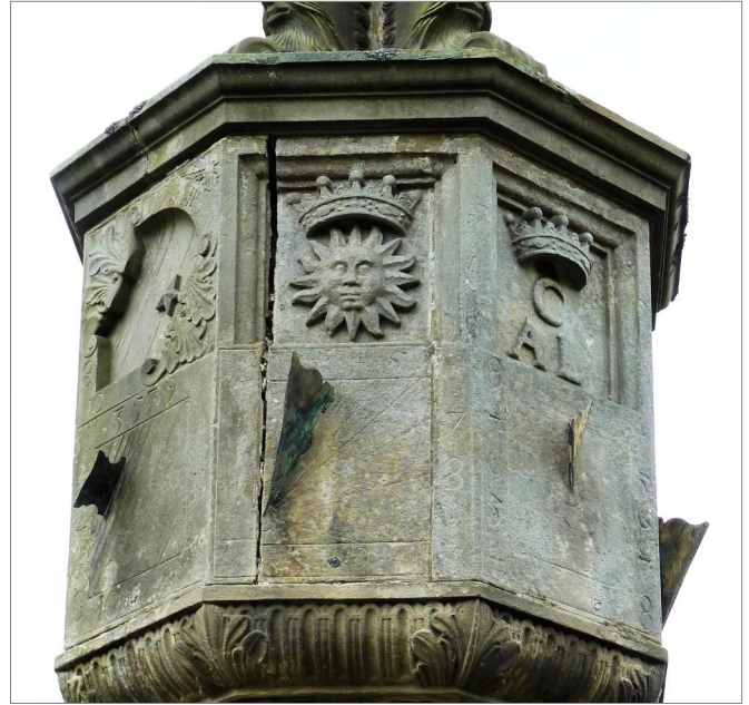
Fig. 10. The north-east face of the Newbattle right-hand sundial and the adjacent north and east faces, with the dials and decorated spaces above them. Again note the huge crack, this time on the north-east face.
