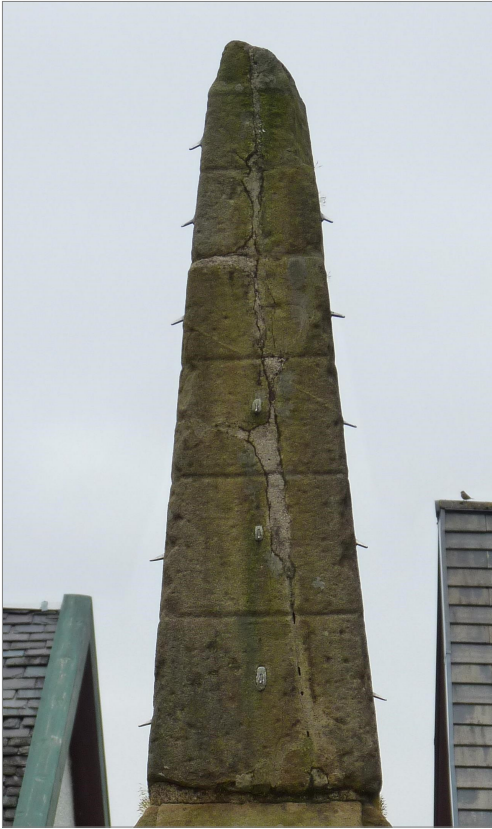
Fig. 10. The serious crack on the finial of the Lochgoilhead obelisk.
