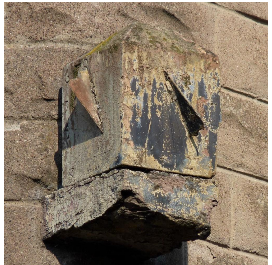
Fig. 6. The north-west and south-west faces of the Melrose sundial. Note the cross patty for noon on the south-west face.
